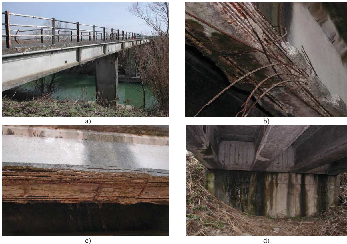
Figure 7: Visual inspection on the bridge: a) General view; b) Corrosion of pre-stressing wires; c) Concrete spalling and reinforcement corrosion; d) Degradation of concrete surfaces.
