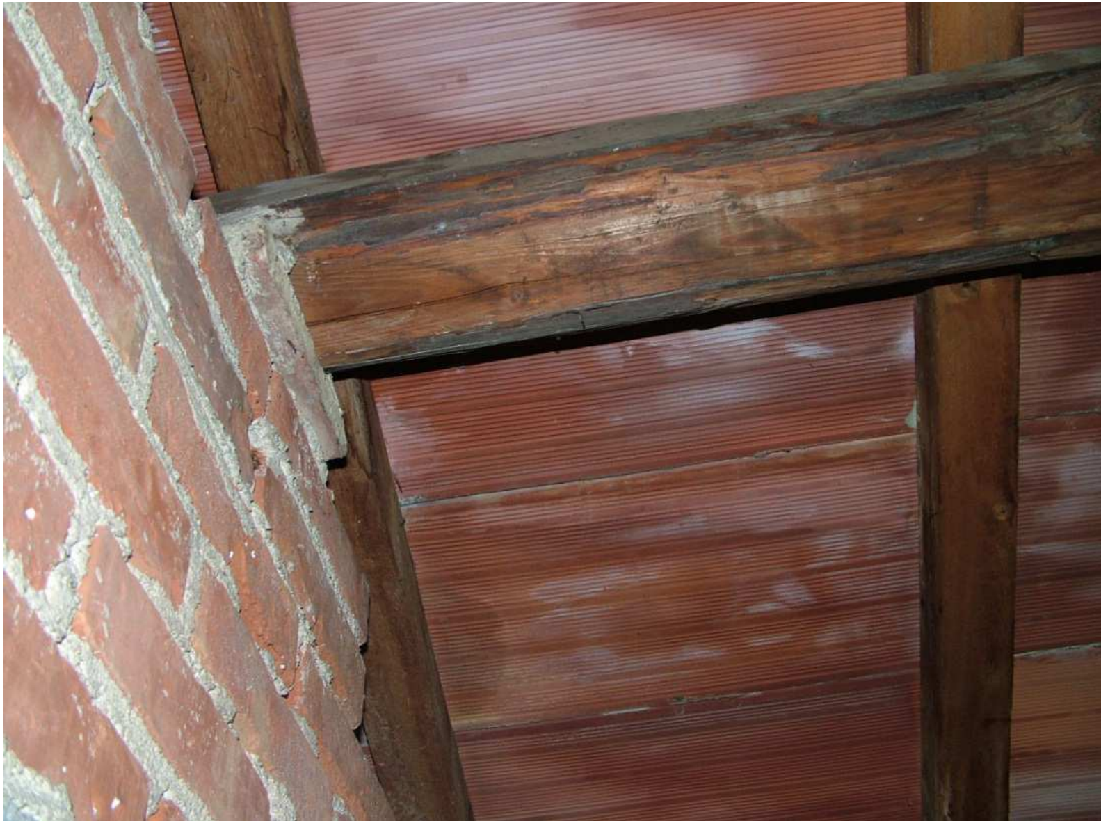
Crack pattern in a beam
