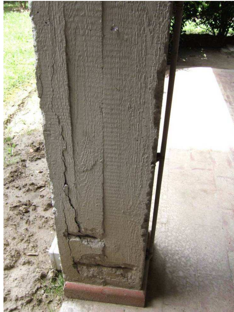
Cracking of concrete cover
