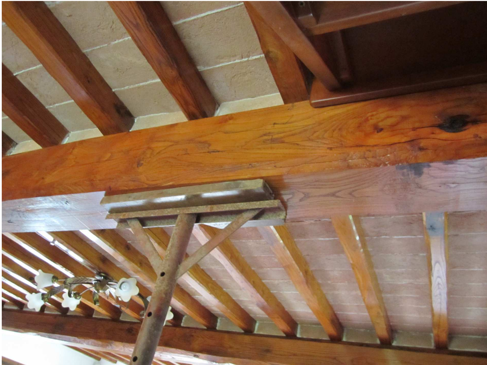
Support and crack
