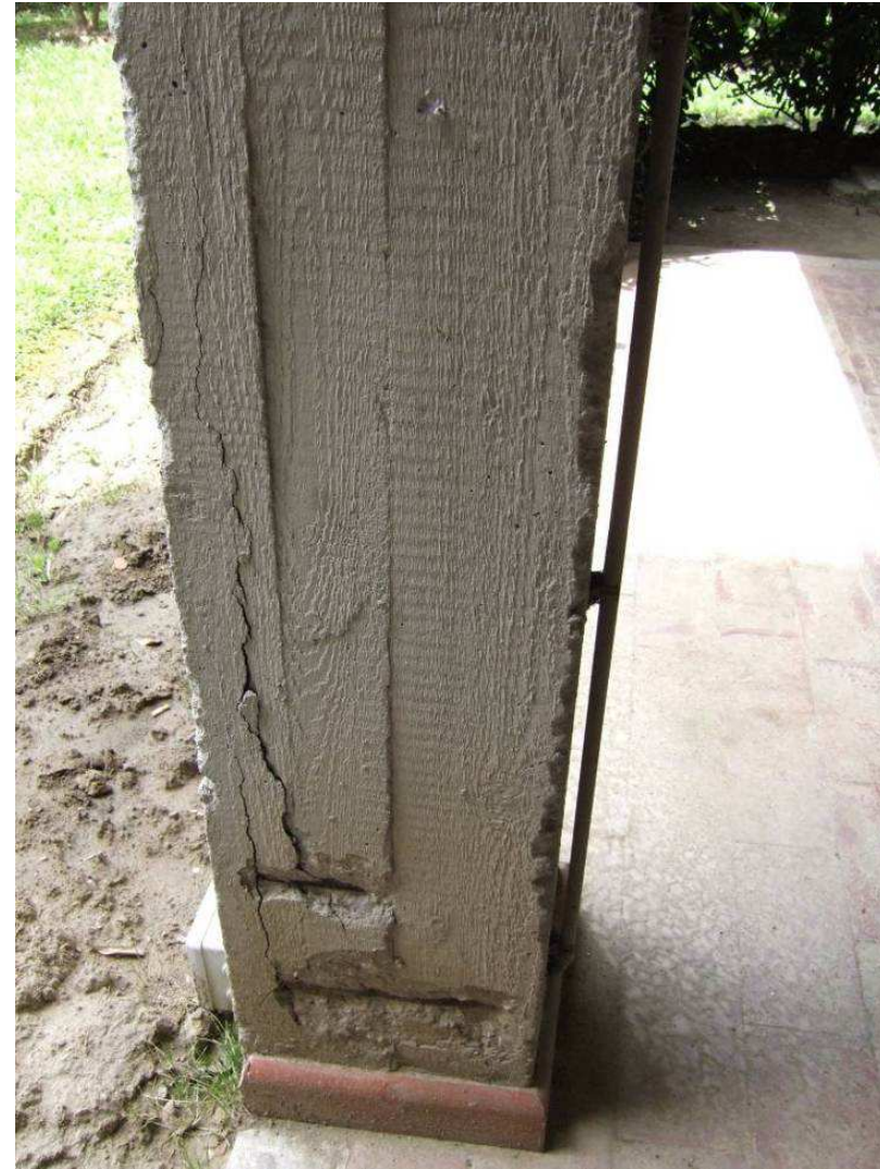
Cracking of concrete cover
